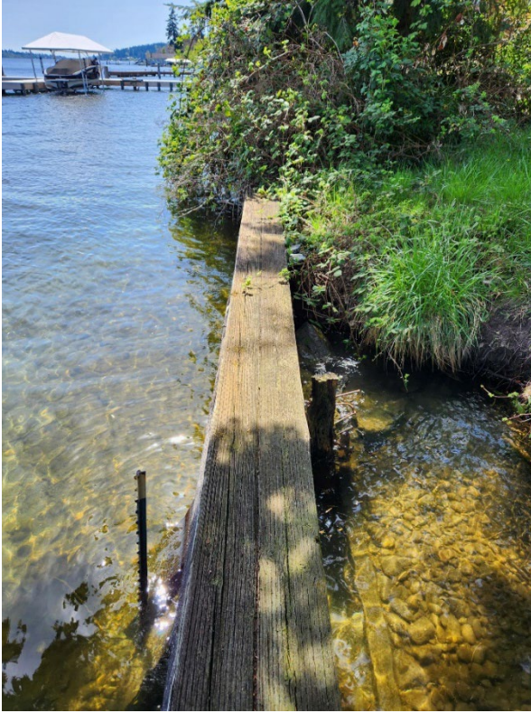
Figure 3. Eroding shoreline behind failing bulkhead.
