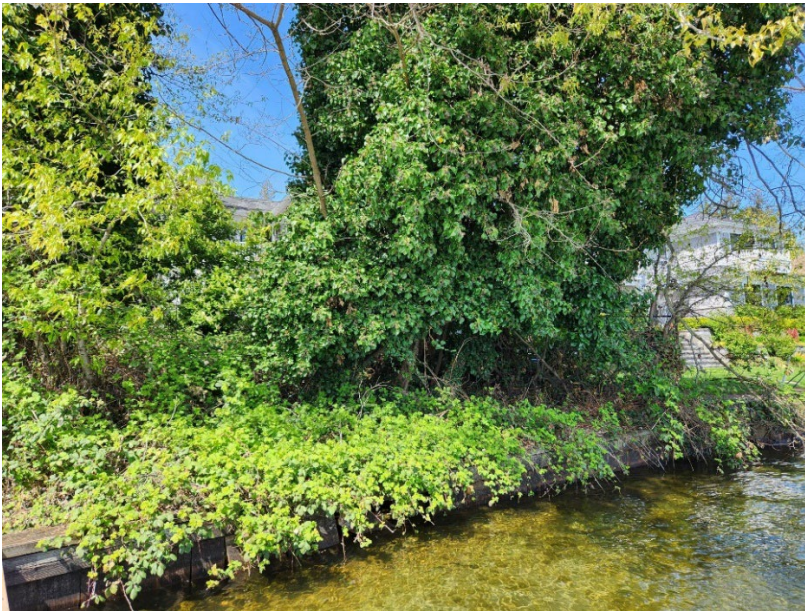
Figure 4. Northern shoreline/bulkhead conditions.
